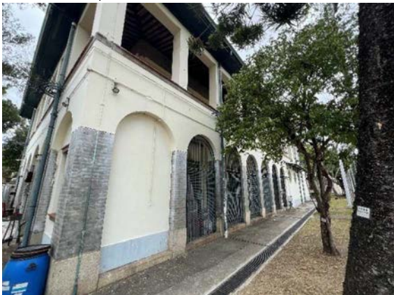
Fig 2.7.10 External walls are painted in a cream finish and jointless grey gauged brick verandah column on G/F.
