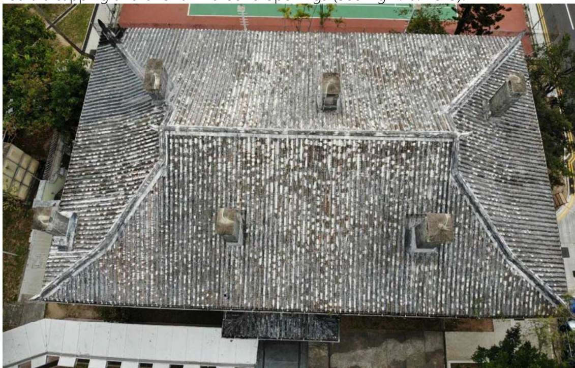
Fig.2.10.1 The roof with the multiple minor repairs and a deteriorating waterproofing membrane.
