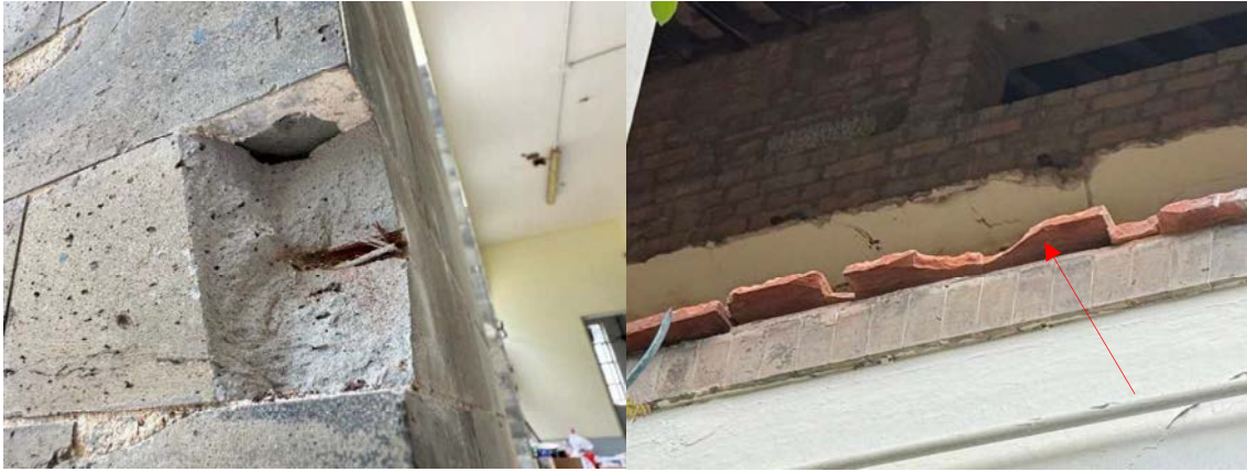
Fig 2.10.2 The broken Jointless Grey Gauged Brickwork. Fig 2.10.3 Broken of the red tile capping.
