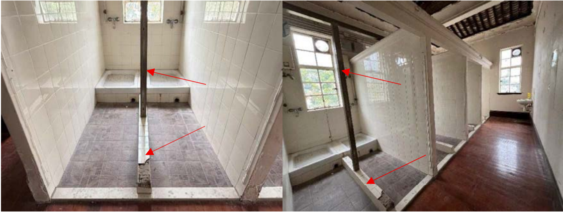
The metall posts and toe walls proposed for demolition are later additions and are considered to have no heritage significance.
