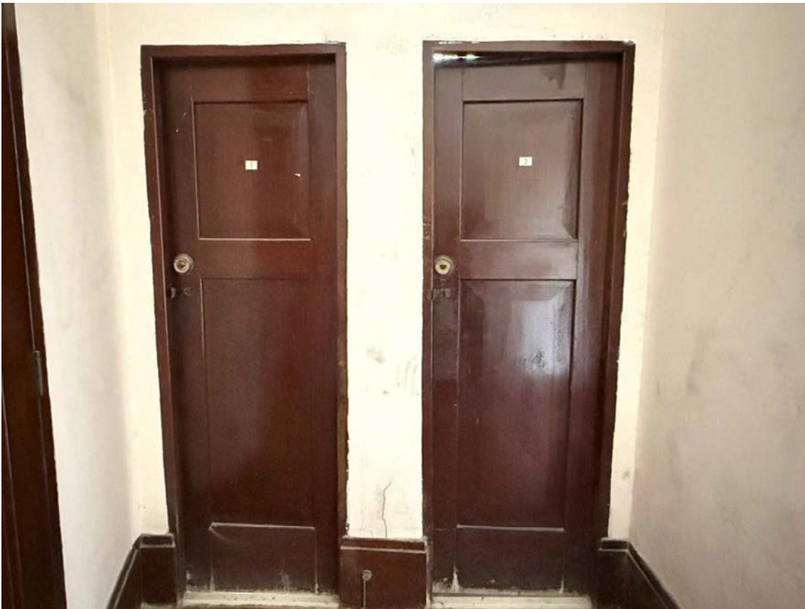
Repair the two original cubicle doors and reuse them in the renovated toilet.
