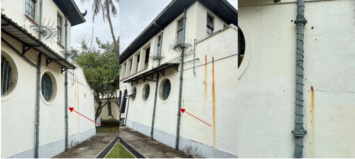
Fig 2.7.16 to 18 The only remaining cast iron rainwater downpipe at Block P.
