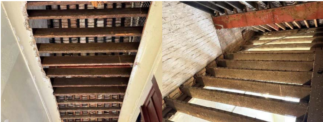
Fig 2.8.24 & 25 The surviving timber ceiling joist above the main staircase on the 1/F.
